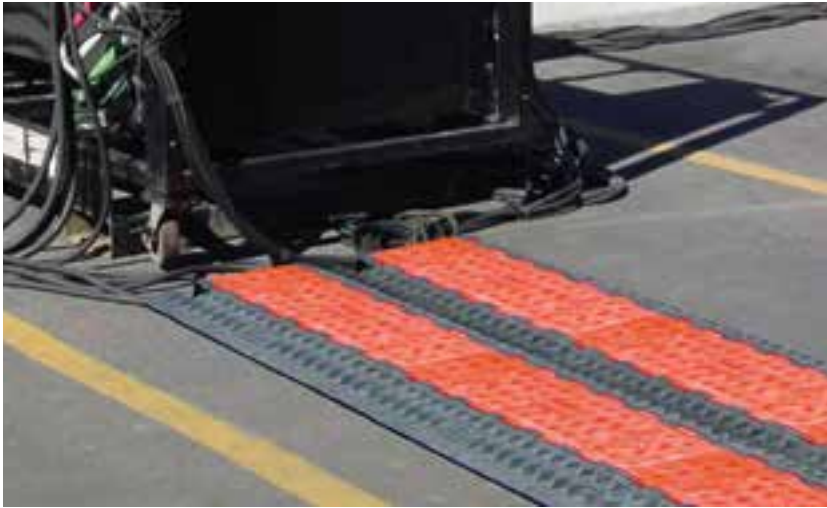
Guard Dogs® in use with a power distribution box
